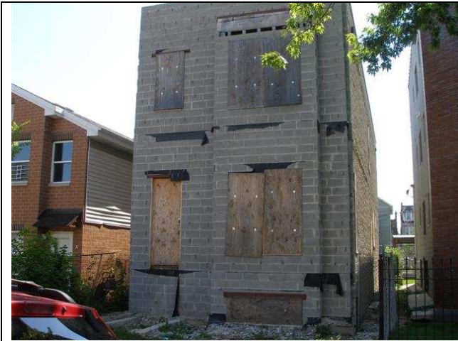
Picture 13. Deterioration of flashing
