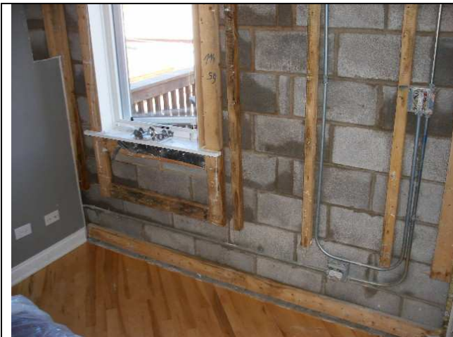
Picture 15. Water intrusion through masonry
