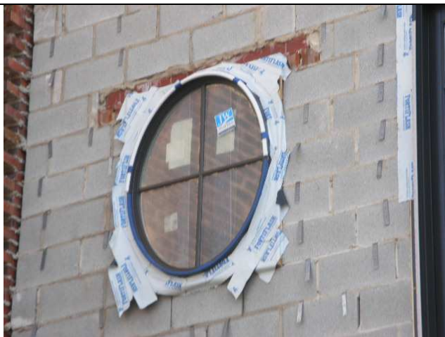
Picture 11. Improper flashing above window
