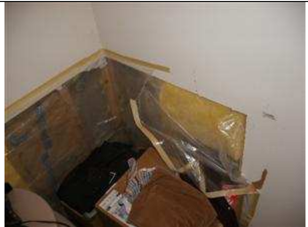
Picture 18. Moisture accumulation in wall
